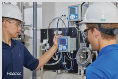
FIGURE 7. Accurate and reliable measurements are critical in a wide range of chemical processing facilities to protect capital assets, ensure product quality, increase process uptime, enhance safety and reduce energy costs
